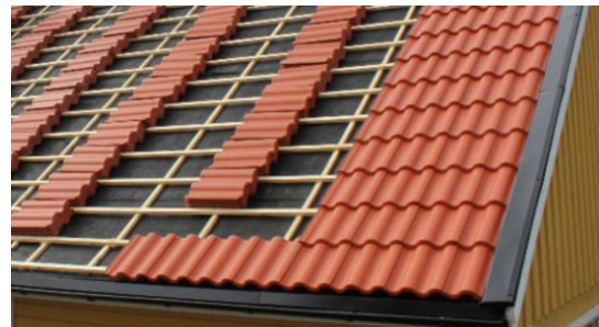
Figure 25. Typical clay tile roof system including a grid of wooden lath and bituminous waterproofing. Photo DW bygg, with permission.
